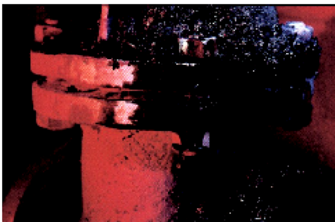
Use of heat transfer fluid with a high vapour pressure can lead to heavy sludge build-up around control valves and pipe flanges.
